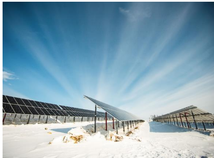
SOLAR POWER PLANT AT SVETLOYE
